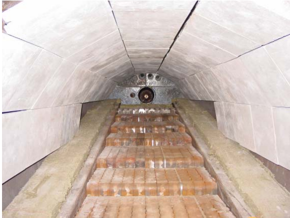
Brennkammer (foto Hollensen Energy A/S)
