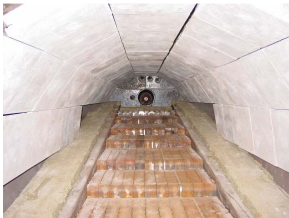
Brennkammer (foto Hollensen Energy A/S)
